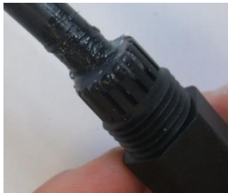
Figure 19 Cable Exit Area
